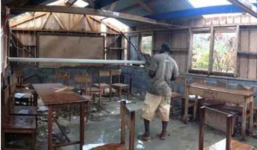
Cyclone Pam caused devastation across many of the 65 inhabited islands of Vanuatu and damaged many schools. (Photo: UNDP) By Andy McElroy
